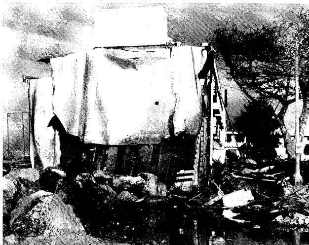
Figure 2. Photo showing collapsed roof section of Portofino Inn, located on Mole B, inside King Harbor, Redondo Beach. Hotel guests were rescued off the roof of the damaged structure by a news helicopter on Sunday evening, 17 January 1988.
