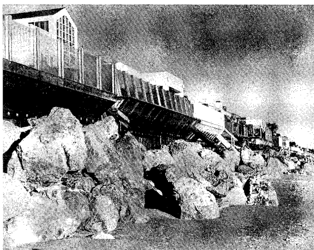
Figure 3. Photo of Malibu Beach showing sand loss and widespread damages to beach access stairs, windscreens and patios. Rock rip-rap protection was placed after 1982-83 winter storm damage.
